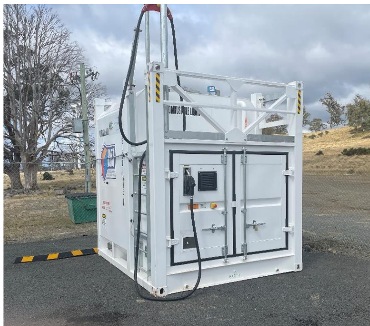
Photograph B6: On-site refuelling system implemented at CHWF in March 2023.
