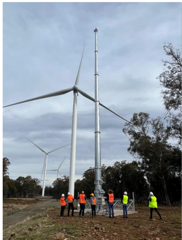
Figure 7.1: EPA and DECCEW representatives inspect IDF-17 during the final stages of commissioning (September 2023).
