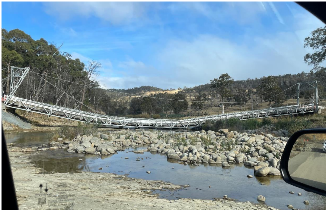
Photograph B6: Waddamana suspension bridge collapses, complicating access to the CHWF at times when the Ouse river is flooded (March 2024)
